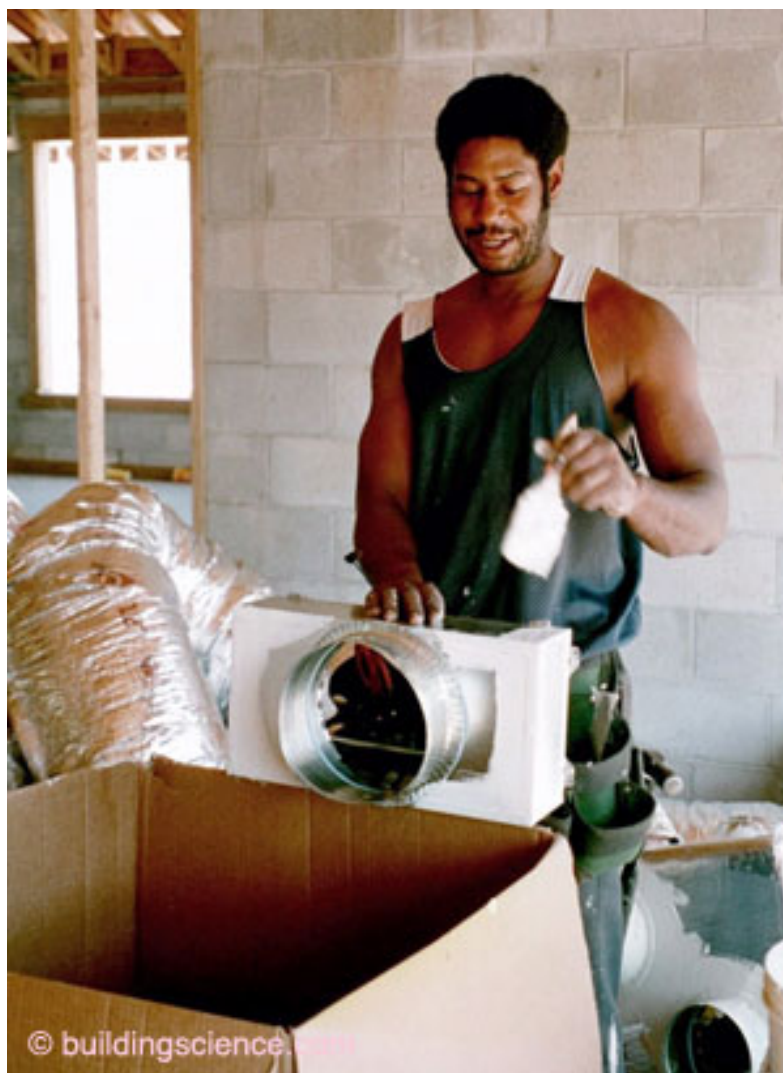
Photograph 1—Mastic Rules: I did not think I would live to see the day where mastic is used to seal all ductwork not just ductwork outside the conditioned space. Woo-hoo!
